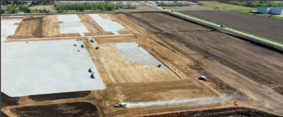
Microsoft Data Center Campus
