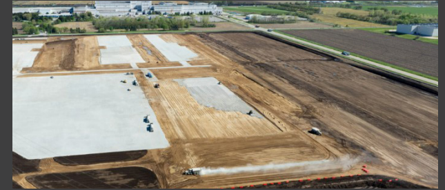
Microsoft Data Center Campus
