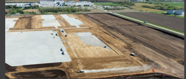
Microsoft Data Center Campus
